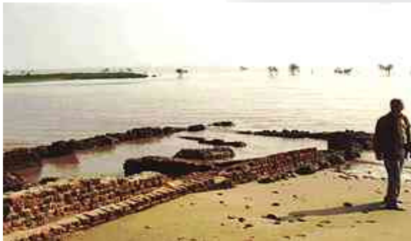
Erosion seen by the exposure of old constructions.
